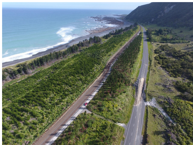
Figure 2. Damage to State Highway 1 and the railway track near Kaikōura (GeoNet, 2016; photo credit Julian Thomson).
